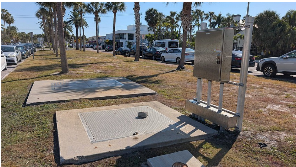
A stormwater pump station on St. Armands. Photo by S.T. Cardinal
